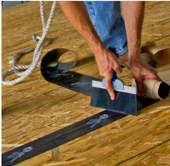
Figure 0-2. Applying qualified tape to roof deck seams using flat blade to eliminate voids and wrinkles.
