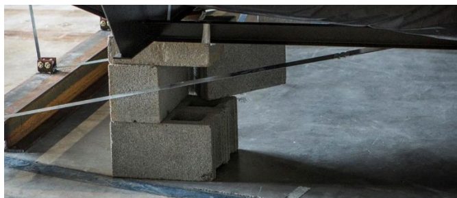
Figure 2.3. Ineligible dry-stack foundation
