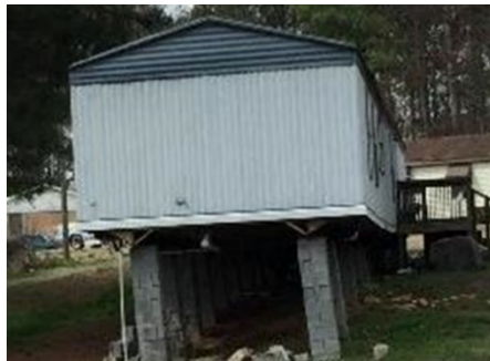
Figure 2.2. Ineligible dry-stack foundation
