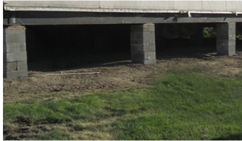
Figure 2.1. Ineligible dry-stack foundation
