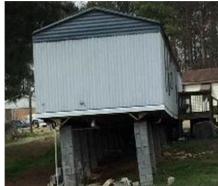
Figure 3. Ineligible dry-stack foundation.
