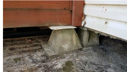
Figure 4. Ineligible dry-stack foundation.
