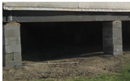
Figure 1. Ineligible dry-stack foundation. No mortar is seen between the blocks.
