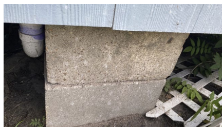
Figure 2. Ineligible dry-stack foundation.
