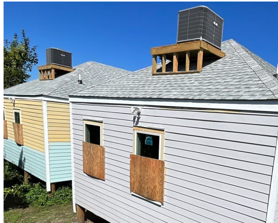
Figure 1: Wood framed supporting platform built over the roof area of a home
