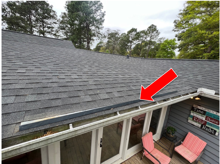
Figure 1: Example of rain diverter installed on asphalt shingle roof.
